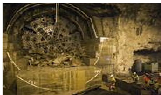
Figure 2: Flooded section of the tunnel due to a lack of geotechnical expertise.
