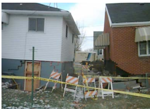
Figure 1: Collapsed foundations and associated cracked mortar within brick and block work of residential structures as a result of unforeseen ground conditions.
